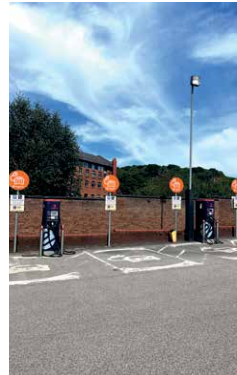
Image above: Electrical Charging Points.
